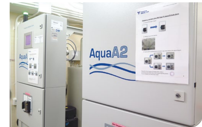
Reverse osmosis water treatment system 淨水處理系統
